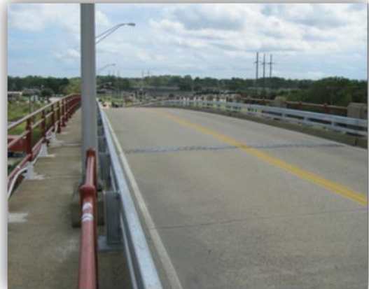
Bridge 2107, Deck and Sidewalk Structural Repairs and Safety Improvements JEB Little Creek-- Fort Story, Virginia Beach, VA
