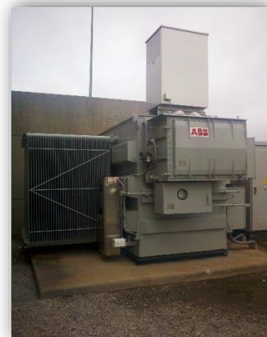
Building A-104 Replace Two Failed Power Distribution Transformers Naval Base Norfolk, VA
